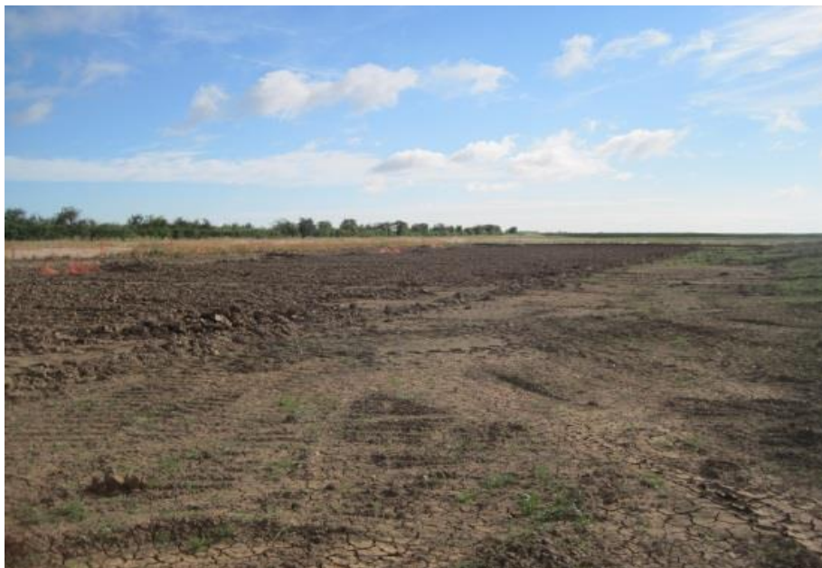
Figure 13: Stripped top soil at Goxhill to enable site establishment and early works
