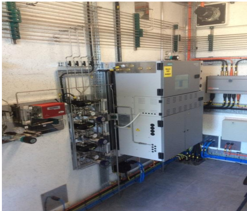
Figure 7: Typical Gas Analyser Installation
